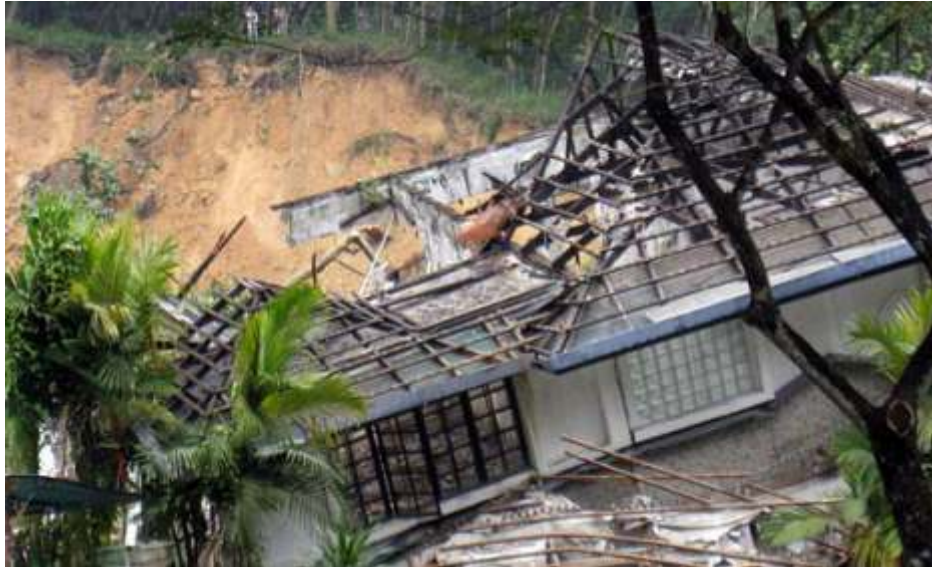
Damage caused by the Bukit Antarabangsa landslide on 6 Dec 2008 (Pic by Raj Kumar)
